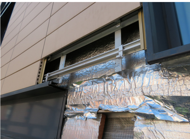
Figure 10: Typical build-up of terracotta rainscreen cladding (note missing cavity barriers around window openings)
